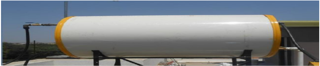
Figure 10- Heated water Storage tank
